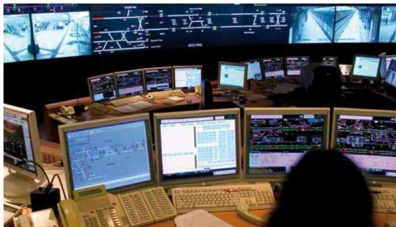
Figure 18: ROCC Type 3 Control Room Example
