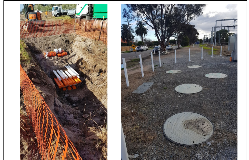
Figure 2a: Typical "Pit & Pipe" CSR during construction, and Figure 2b: typical CSR main route pit array with posts as errant vehicle protection – as adjacent to a suburban road.
