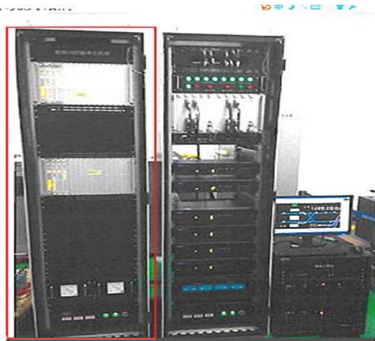
Station interlocking machine
