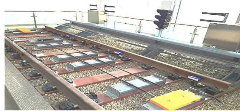
Train-ground communication equipment
