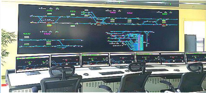
Central TIAS equipment
