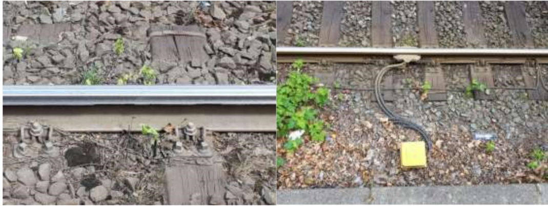
Figure 10. Track condition of section 208 and 210 [3].
