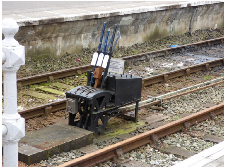
Figure 4. A typical three lever Mechanical Ground Frame
